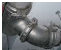
SS 304 potable water line
