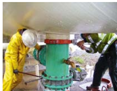
Water Treatment, USA
