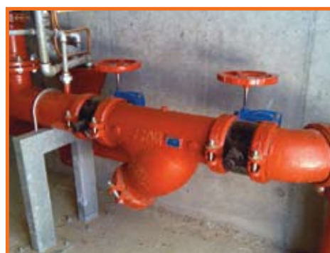
Edipower 800 – Power Plant, Italy
